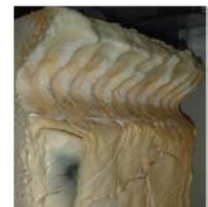
Accelerated refractory wear at metal line due to corrosive nature of foam
